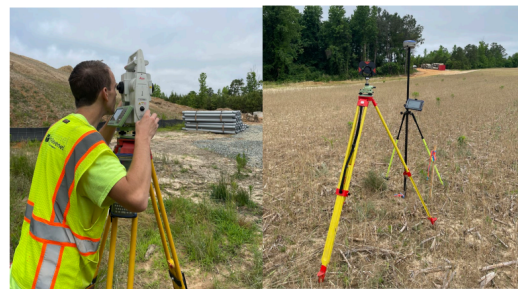
Figure 3: Total station operation (left), Back-site (right image shown on a yellow tripod), GPS shown on right image as black pole with tablet and round antenna
